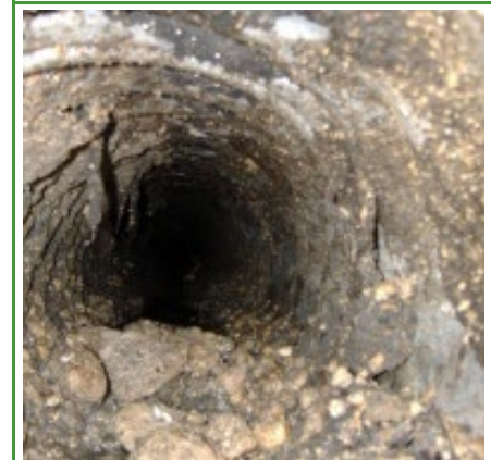
Initial investigation of grease management (top), grease build-up catch basin sump (middle), and grease build up in pipes found during video inspection (bottom). Photo Credit: Dan Smith (City of Federal Way)
